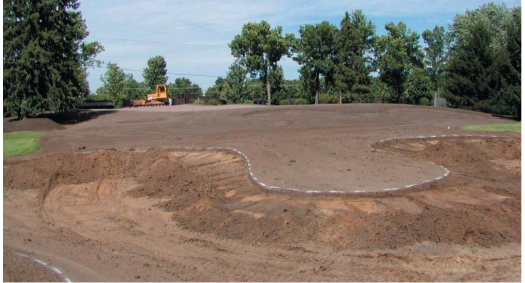
Hole 12 fairway bunkers and green after completion of final shaping and bunker edging.
